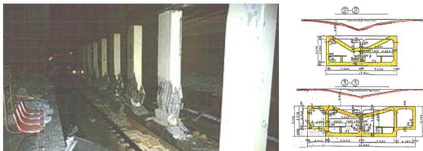
Figure 7-1. Collapse of Dakai tube station
